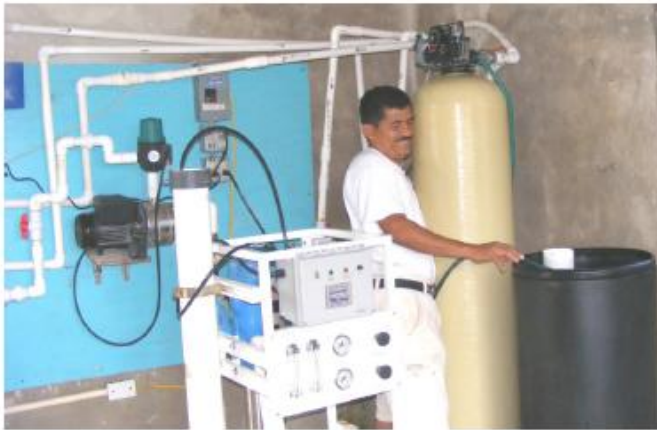
VIM Director, Isaac, operates the repaired water purification system.
